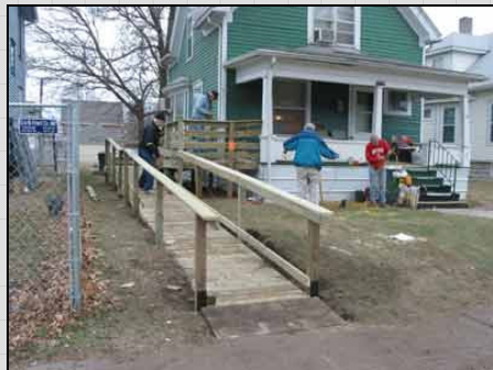
Wheel chair ramp designed by John Wauer and built by RCRV members for Aging Services
