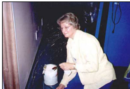
Painting the walls of the day care room of the Heart of Iowa
